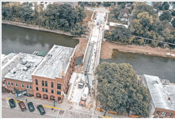
An ariel view of the Keystone Bridge Project that is expected to be finished by the end of 2023.
