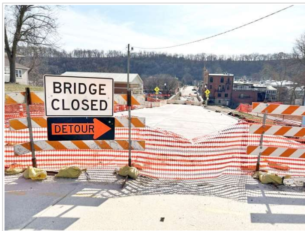
Elkader's Keystone Bridge project is scheduled to resume this week. Work is still expected to be completed by Dec. 28 of this year. (Photo by Willis Patenaude)
