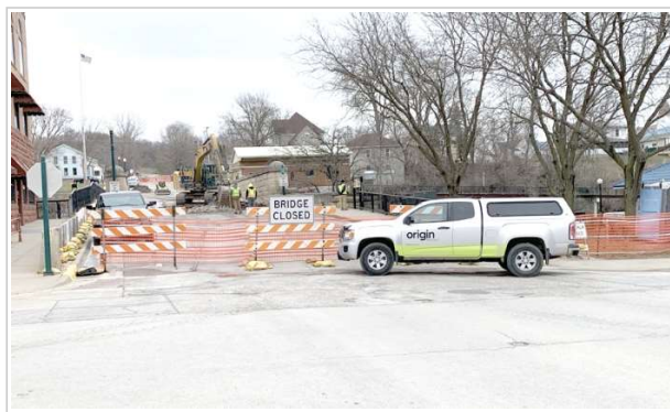
Elkader's Keystone Bridge rehab project came to a sudden halt April 20, after a widening crack was discovered. The find shut down not only construction but pedestrian access across the bridge, out of caution. (Times-Register file photo)
